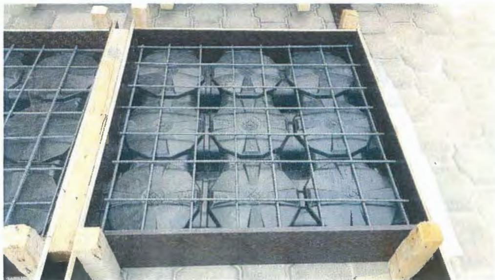
Figure 3: ABS disposable formwork with mesh steel reinforcement prior to concrete casting for sample Group (II) [normal concrete] and Group (III) [fiber concrete].
